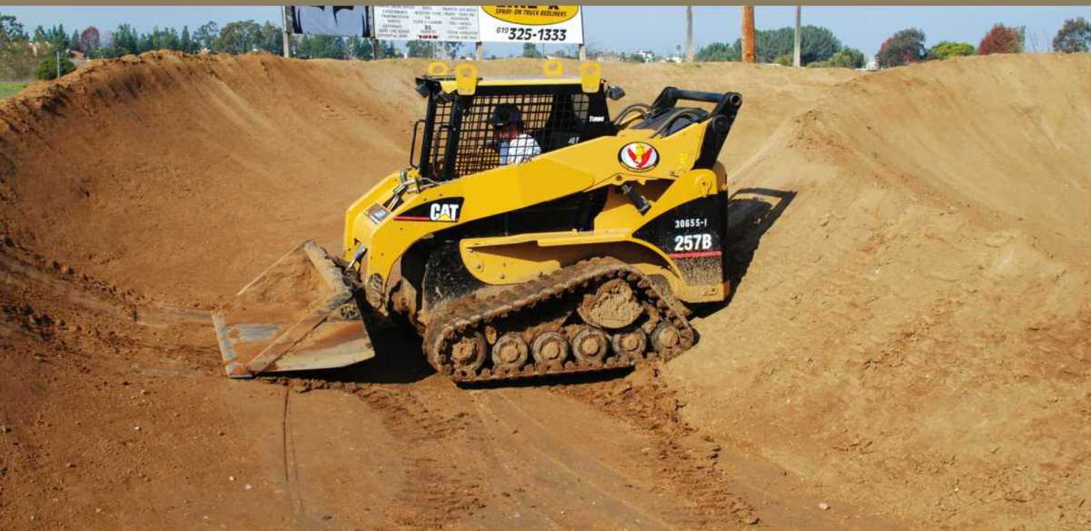
Below: Jacob McCurdy uses a Cat 257B to shape the banks and slopes at Kearny Moto Park.
