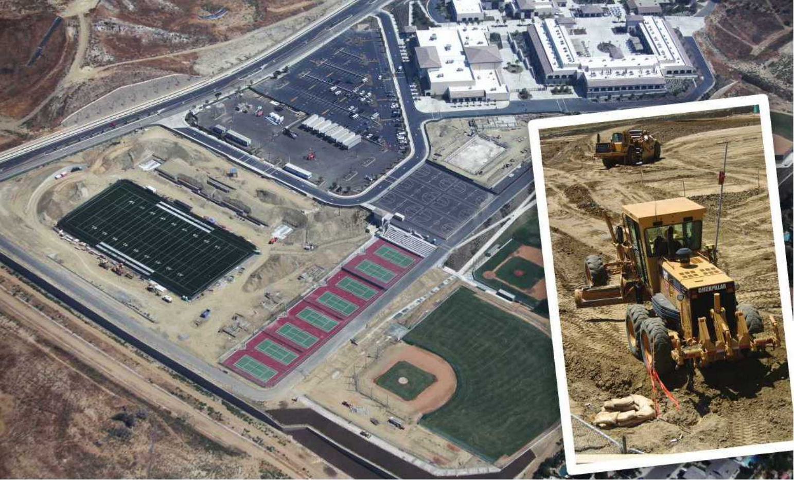
(Above Inset) Byrom-Davey, Inc. relies on companies like Heavy Equipment Rentals for their heavy equipment needs. They rented several machines from Heavy Equipment Rentals for use on the Yorba Linda High School Sports Complex including: scrapers, dozers, wheel loaders and excavators. (Above Main Photo) Aerial shot of Yorba Linda High School.
