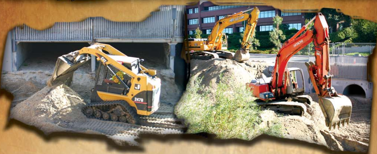
(Above Left) Ryan Monteleone Excavation, Inc.'s Cat 247 track skid steer. (Right) Ryan Monteleone operating his Hitachi EC200 excavator.
